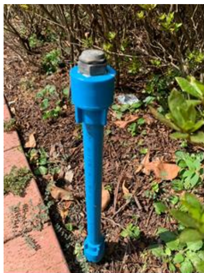
Fig. 1 The water pipes that connect the nozzles on the ground surface must be high density polyethylene pipes or soft plastic pipes of the same quality. An adjustable 180° brass nozzle should be installed in every 3 metres and the plastic pipe should be 30 cm above the soil surface.
