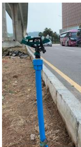
Fig. 2 In a large area or corner, a movable sprinkler nozzle with adjustable angles should be installed.
